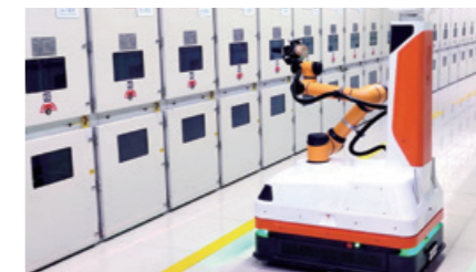
High-voltage distribution cabinet operation
